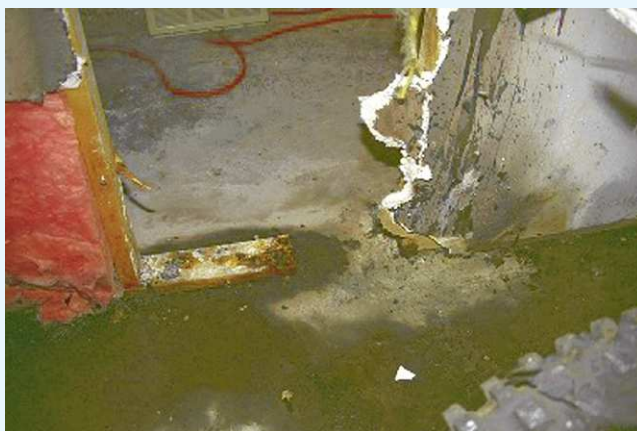
Figure CS12.2.2 Close-up view of the hole in the wall made by the fire department as viewed from the garage side.
