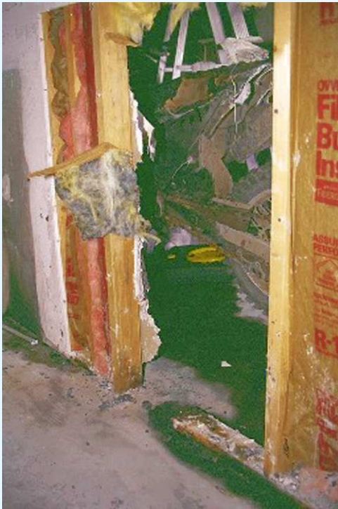
Figure CS12.2.3 View of the same hole in the wall as viewed from the utility room side. Note the defect in the wall where the sill plate is missing.
