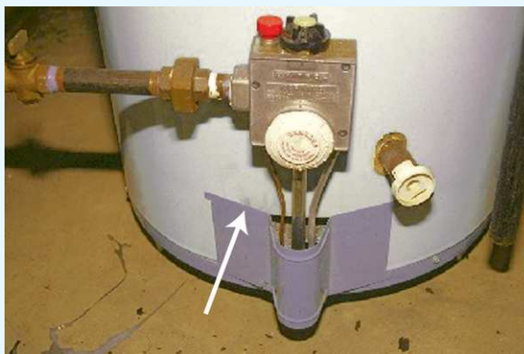
Figure CS12.2.5 Close-up view of the base of the water heater. The arrow indicates the soot mark caused by the ignition of the gasoline fumes by the burner of the water heater.
