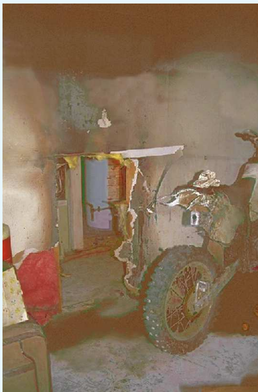
Figure CS12.2.1 Overall view of the point of origin from the garage side showing the location of the motorcycle in relation to the hole in the wall.
