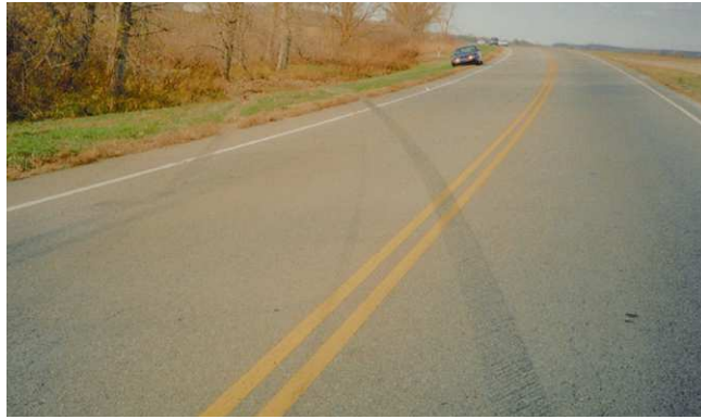
Figure 18.6 Skid pattern showing car was rotating counterclockwise as it crossed over to the oncoming side and struck a tree.
