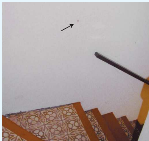
Figure CS5.2.1 Scene photograph of shooting. Defect in wall above and to the left of banister is from a projectile.
