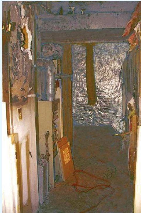
Figure CS12.2.4 View into the utility room showing the water heater and furnace on the left and the hole in the wall on the right.
