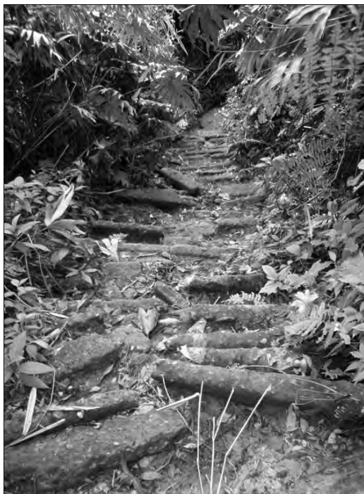
Figure 8.2 Broken and poorly maintained concrete steps on the descending trail
