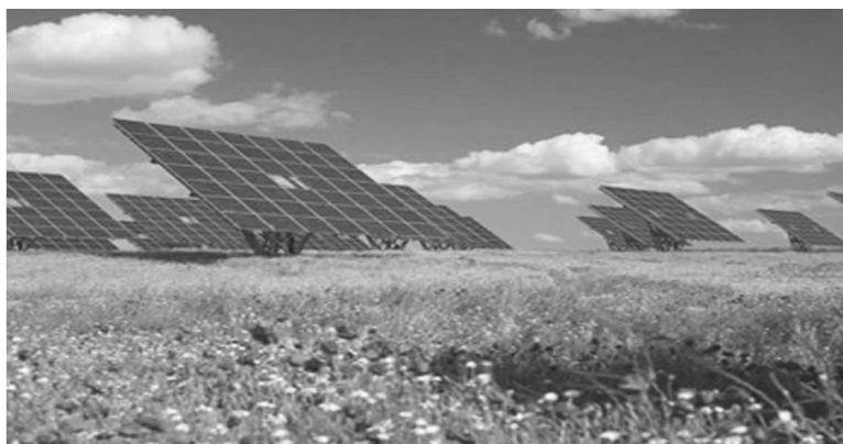
Fig. 16.2. Solar photovoltaic (PV) panels providing green energy for agricultural growth.
