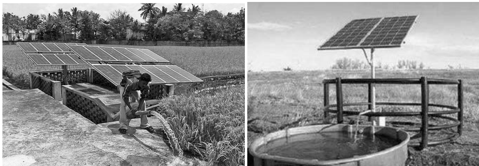
Fig 16.5. PV integrated water pumping application
