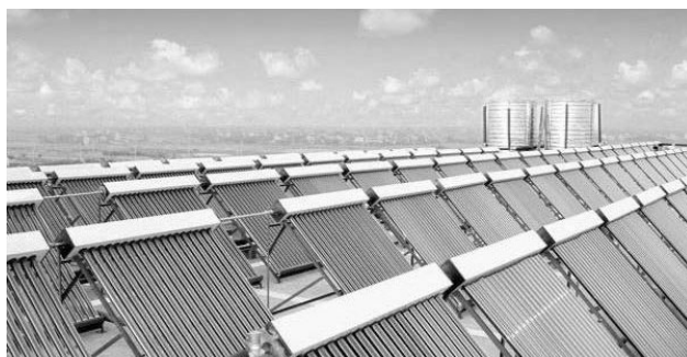
Fig. 16.11. Solar water heating system
