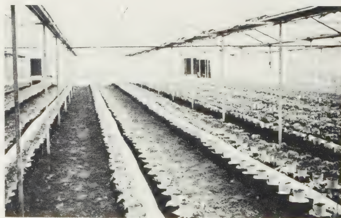
Fig. 23.8 Ducted warm-air heating system with a duct between each double row of plants. (photo B. R. Smith)
