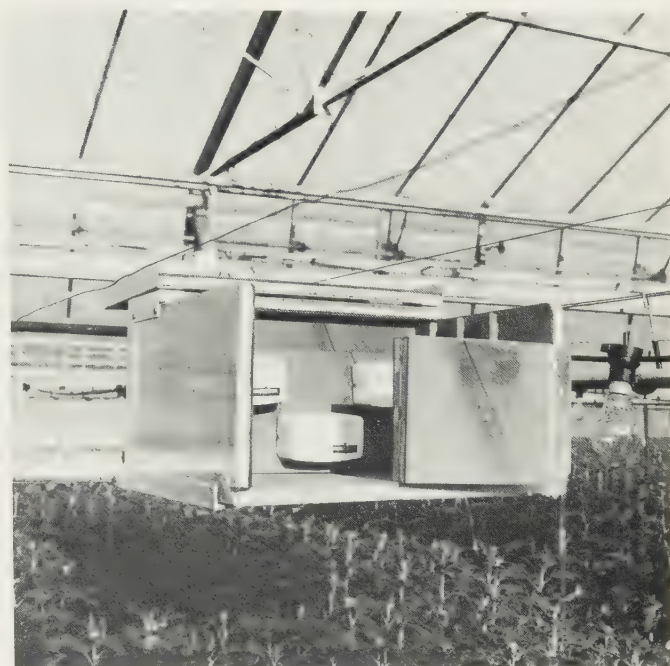
Fig. 23.12 Silsoe Research Institute-type aspirated thermostat. ( Electricity Council )
