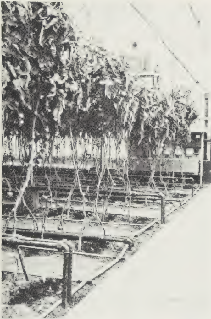
Fig. 23.7 Pipework for high-speed hot water heating system. A loop of 32 mm pipe is provided for each double row of tomatoes, the pipes of alternate loops being supported on the concrete dollies on which roof supports are mounted. The aspirated-screen thermostat and the irrigation pipes are also shown. (photo B. R. Smith)
