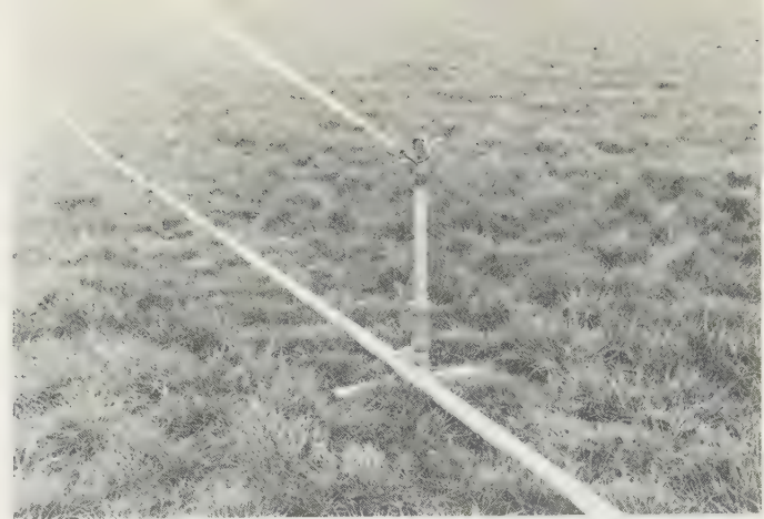
Fig. 10.9 Self-sealing bayonet-type standpipe coupler to facilitate moving of sprinklers. (Wright Rain)
