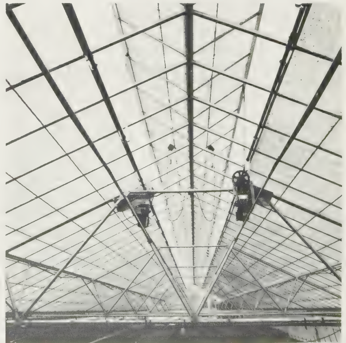
Fig. 23.9 Ridge-vent motors and limit switches in a wide-span glasshouse. ( Electricity Council )
