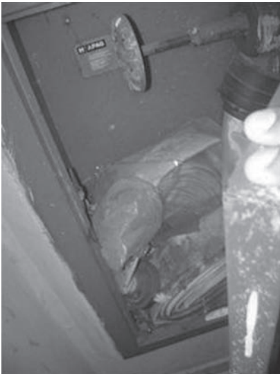
Figure 1. Hydrant disabled accumulating the garbage.
