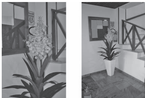
Figure 6. Extinguishers hidden and obstructed by flowers.
