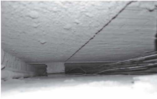
Figure 1. LPG ventilation and electrical cables at the same pipe.
