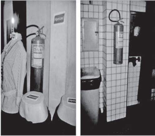
Figure 3. Extinguishers without any identification and obstructed by goods.
