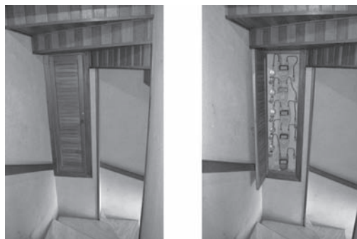
Figure 10. LPG cabinet counters inside stair. Ceiling composed of combustible material. Intermediate landing with tapered steps.
