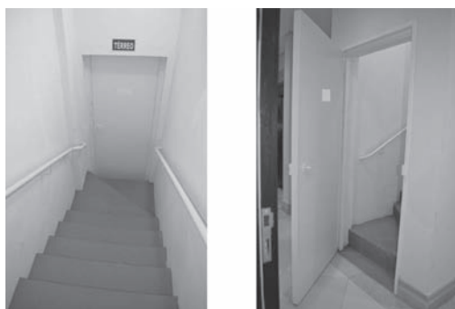
Figure 7. Enclosed stair with tapered steps. Improper encapsulation.
