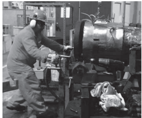
Figure 8. MMH—pulling coke barrel—(maintenance activity).
