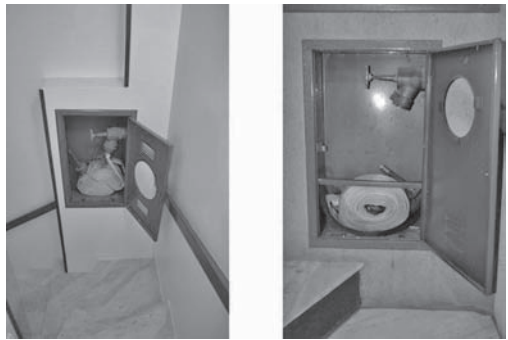
Figure 4. Hydrant inside enclosed stair. Fire hose tied up and with expired inspection term.
