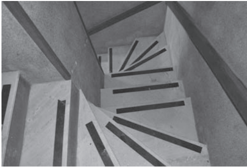
Figure 2. Handrail on one side only of the stair. Intermediate landing with tapered steps. Improper width scaling—minimum width less than 1.05 m.
