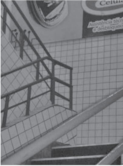
Figure 2. Stairs without emergency lighting.
