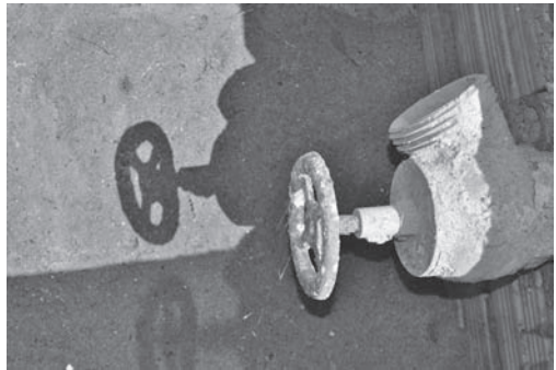
Figure 5. Hydrant Registry closed—cement embedded and in a condition that prevents the hose coupling, making it impossible to use.
