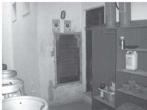
Figure 9. LPG central confined under the ramp to the second floor, extinguishers removed and placed improperly to install the electric drive motor pump set; storage of flammable chemicals (solvent).
